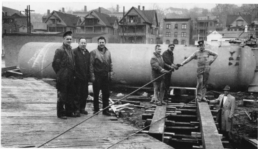
In the process of loading one of the 35-ton propane tanks onto a flat car are (left to right) Charles Lewis, Vincent Valuckas, Humbert Mucci, George King, Henry Yeske, Ernest Garbauskas and Charles Dubuque, foreman.
